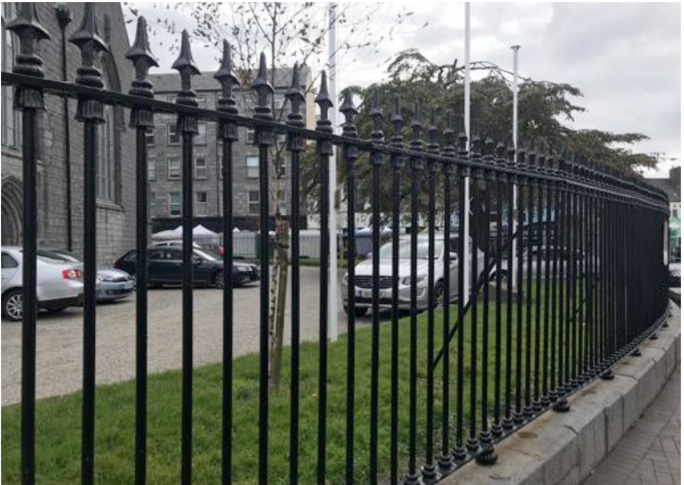
Conservation and painting to 53 metre length between main gates and Lynch's Window
